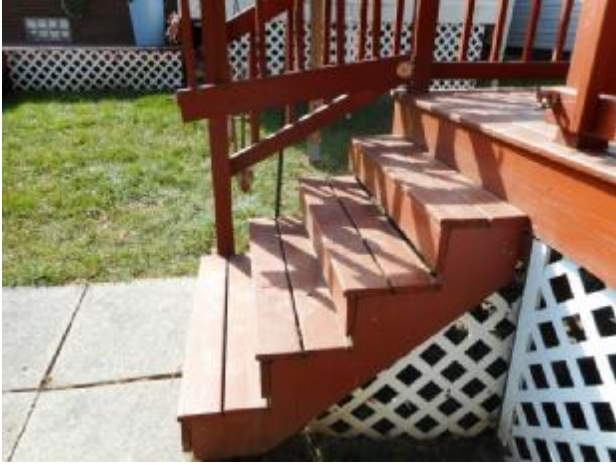
Lacking proper railing
